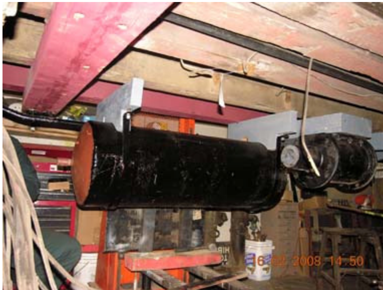
Auxiliary reservoir no. 1 and brake cylinder mounted under 100.
