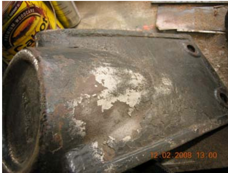
Pole pocket showing aluminium paint under the black.
