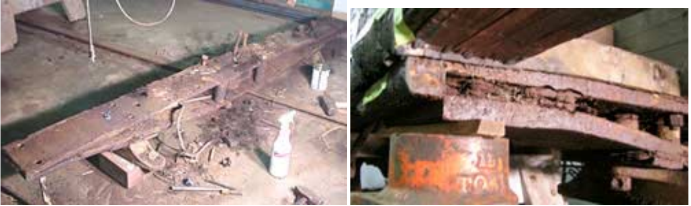
Bolster after removal Build-up of corrosion between upper and lower plates Note the bent-over upper plate.
