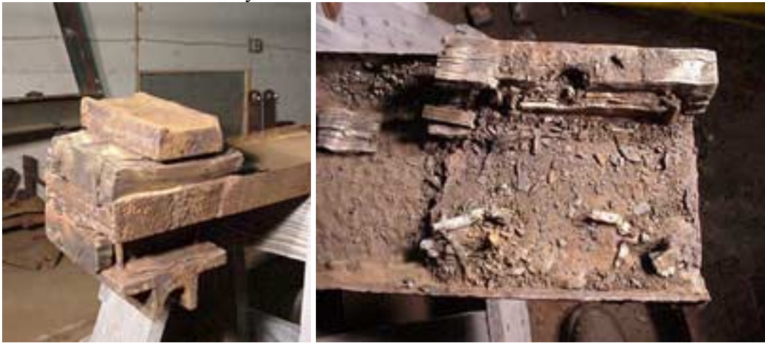
Spring plank (the channel), spring seat, spacer blocks and lower casting for swing link pin. Rusted area after removing block. Stubs of lag screws showing.
